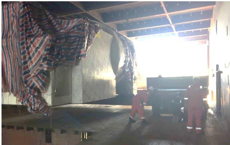
figure 3-28 positioning tank over opening at deck 3 showing cradle and removal of SPMT's
